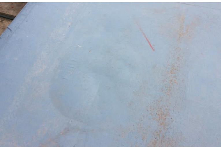
Blisters caused by moisture retention from a wet deck.
