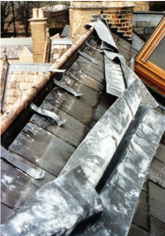
Ridge flashings blown off due to incorrect clips.
