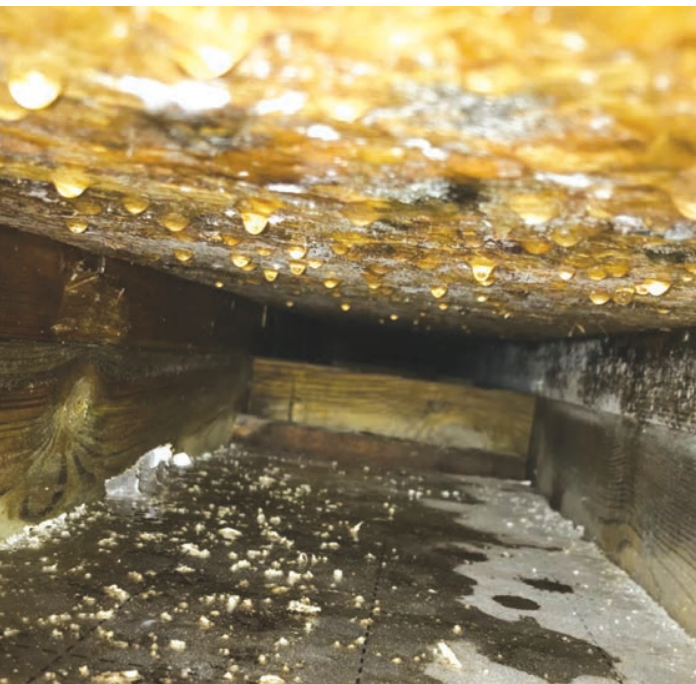
Interstitial condensation used to be considered acceptable periodically in the winter, but not for sustained, long periods, otherwise mould could set in.
