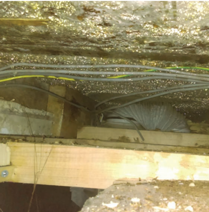
When the perfect conditions come together, i.e. high moisture and low external temperatures, interstitial condensation occurs.
