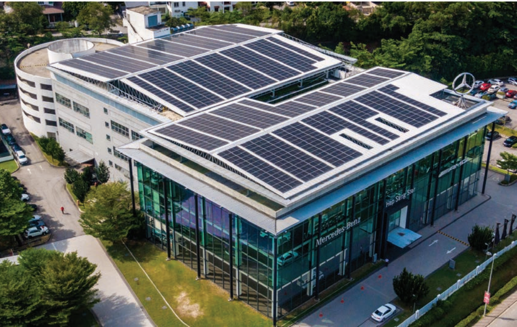
Hap Seng Star is the main distributor of Mercedes-Benz's vehicles in Malaysia. In order to meet their sustainable development goals and save operational costs, a 1.7 MW PV system was installed, saving 73,541 kg of carbon dioxide, equivalent to taking off the road 15.8 cars for a year.
